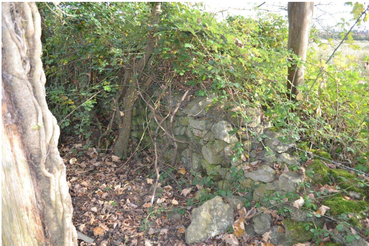
Plate 42: Drystone wall forming part of the western limb of the physical enclosure defining the strip of woodland along the western edge of Field 4 (Gaz. 24).
